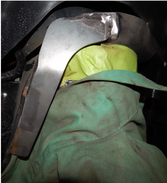
Gusset shown welded on driver's side spring bucket.
