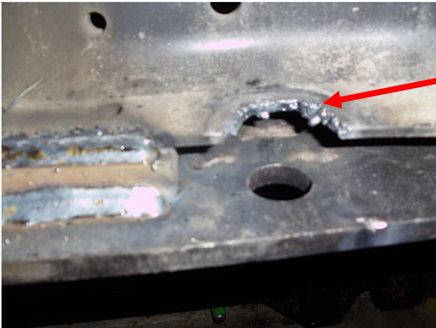
If the factory cross member covers up the air bag hole, use a torch to make clearance.
